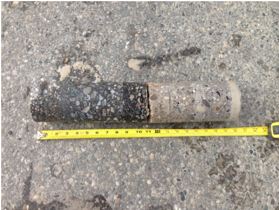
Core Photograph No. 6: 10-1/2 inches of Bituminous Concrete 8-1/2 inches of Portland Cement Concrete
