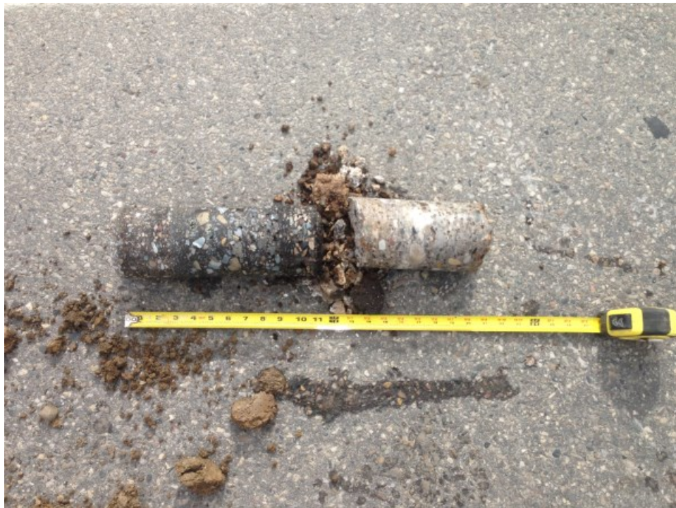
Core Photograph No. 8: 12 inches of Bituminous Concrete 8 inches of Portland Cement Concrete
