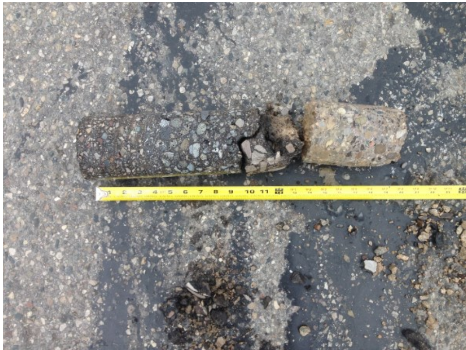
Core Photograph No. 10: 13 inches of Bituminous Concrete 7 inches of Portland Cement Concrete
