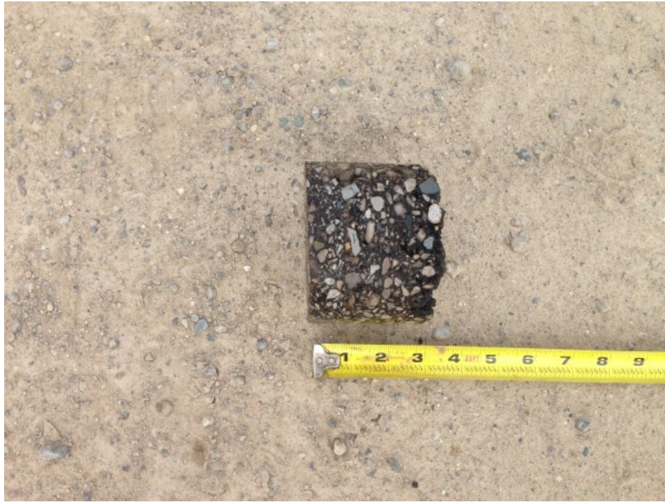
Core Photograph No. 11: 3 inches of Bituminous Concrete 9 inches of Portland Cement Concrete (Fractured)
